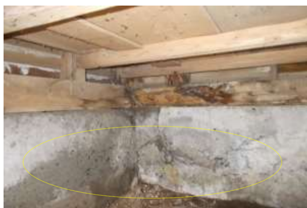
洋室床下腐朽
